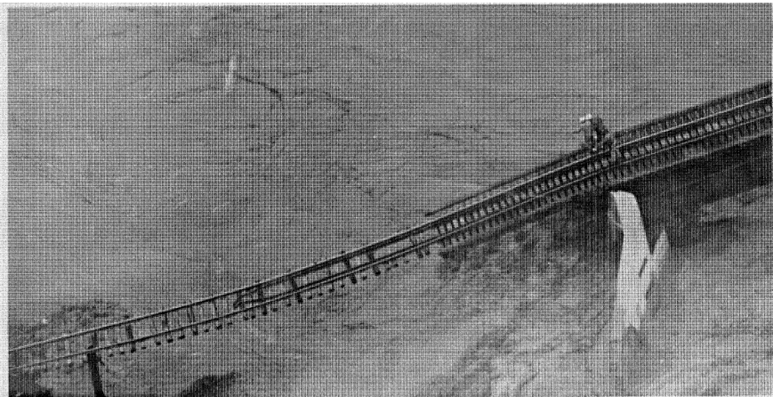
WATINO NAR LINK CUT — Northern Alberta Railway engineers take a precarious look at the ruins of the Watino span over the Little Smoky River, which ripped out the bridge and closed highway traffic late Tuesday. Minutes after this photo was taken, the sup-
