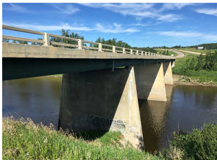
Looking across the river from the right bank at the downstream side of the bridge
