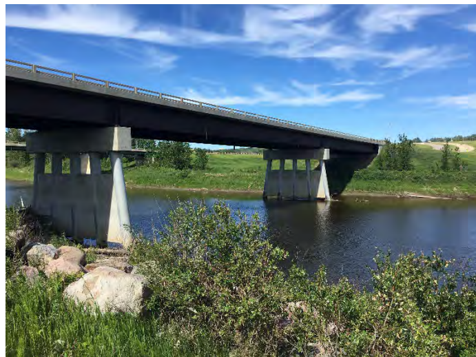
Looking across the river from the right bank at the downstream side of the bridge
