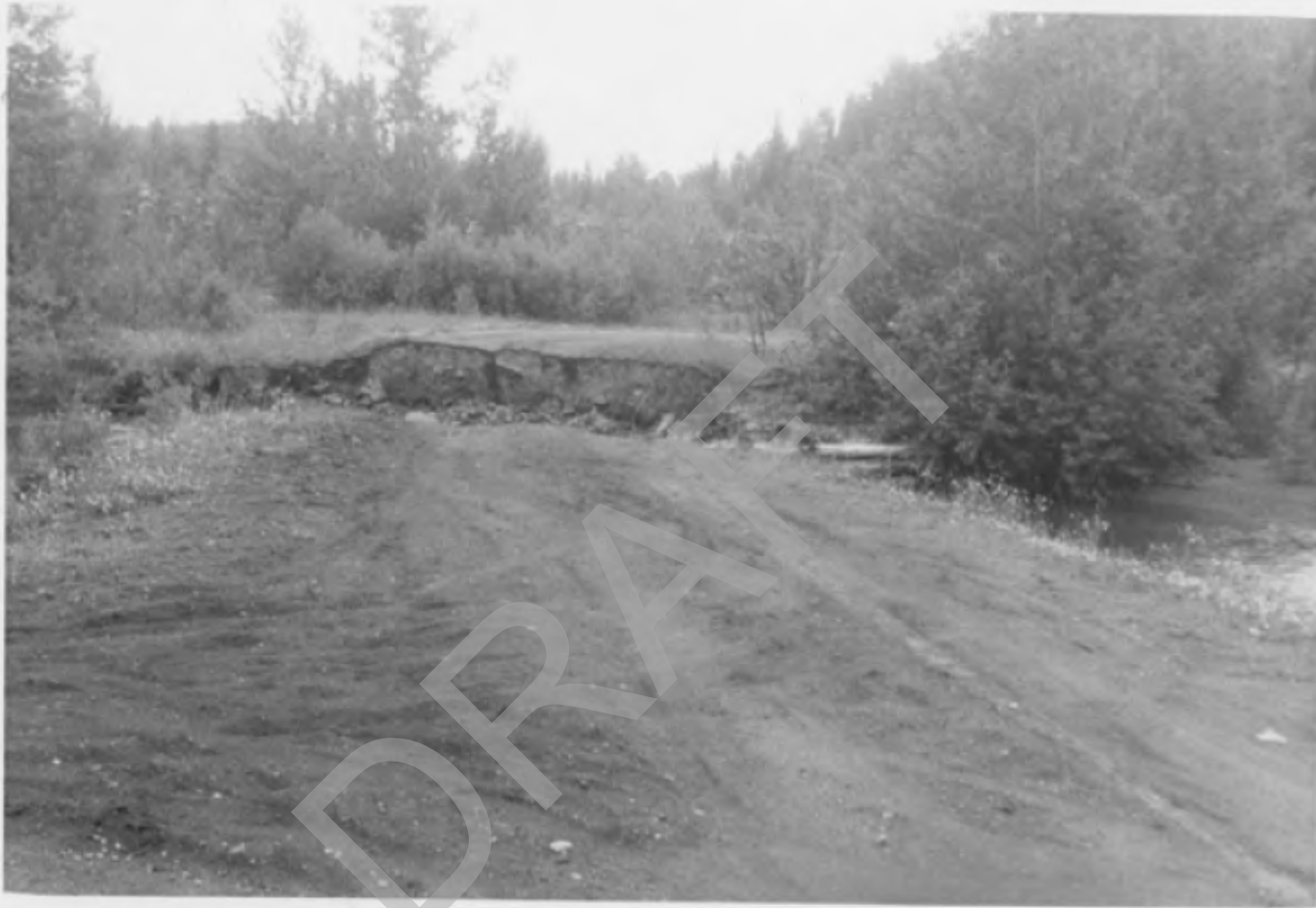
Notes: a) West Side, looking north. Old Embarras Drive Bridge completely washed out. (photo obtained from TEC bridge file #76138 flood documentation).
