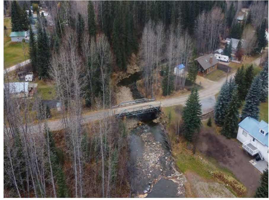
4) Aerial view looking downstream on Embarras River at Embarras Drive Bridge near PXS-54.
