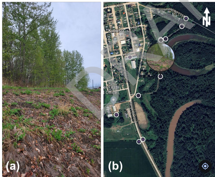
Figure 3 Berm at Kinuso. a) Standing on the Berm Toe and Viewing NW, b) Location of Picture in (a)
