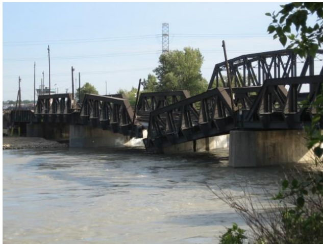
Photo 13: Collapsed CP Rail Bridge at Bonnybrook after rail cars were removed on July 10, 2013 (Provided by the City of Calgary)
