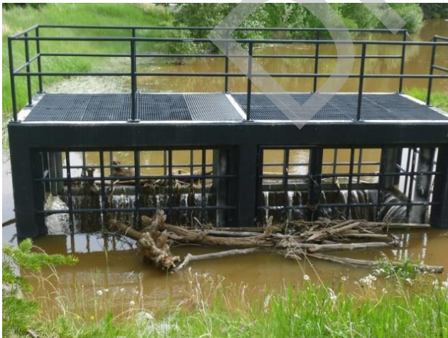
Photo 9: Drop-Inlet Structure at Lott Creek Drive on June 23, 2013 (Provided by the Elbow Valley Residents Club)
