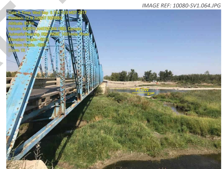
2. View looking across the river from right bank at the bridge abutment.
