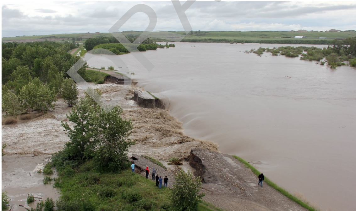
Photo Source: "Carseland Bow River Headworks: Repair of Fuse Plug at Johnson's Island" (AMEC, March 2014)
