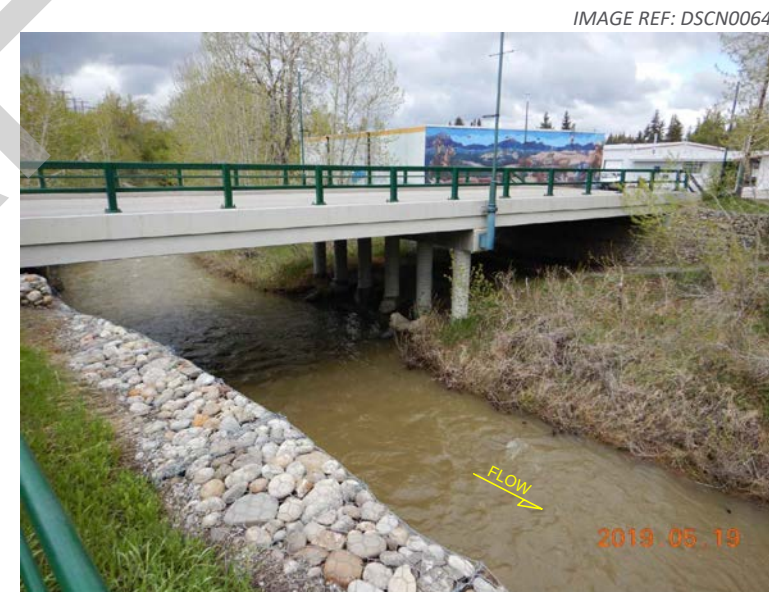
2. View looking obliquely upstream across the creek from the top of the right bank revetment.
