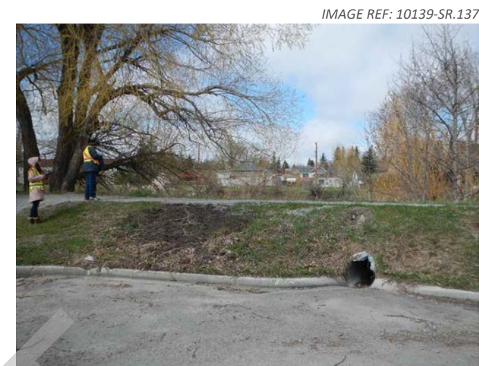
1. View looking at the upstream end of the berm toward the creek (on the other side of the flood control structure). Flow on the creek is from left to right. The corrugated steel pipe culvert that passes through the berm is not equipped with a flap gate to prevent floodwater from flowing toward the street (Church Avenue).
