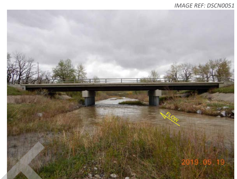
1. View looking downstream from the island in the middle of the creek.
