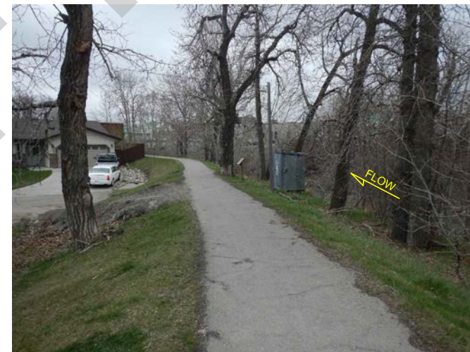
2. View looking downstream along the berm at the south end of Morden Avenue and at the location of the Water Survey of Canada hydrometric station (WSC 05AA004) on Pincher Creek. A corrugated steel pipe culvert passes through the berm near the end of the driveway and is not equipped with a flap gate to prevent floodwater from flowing toward the street.
