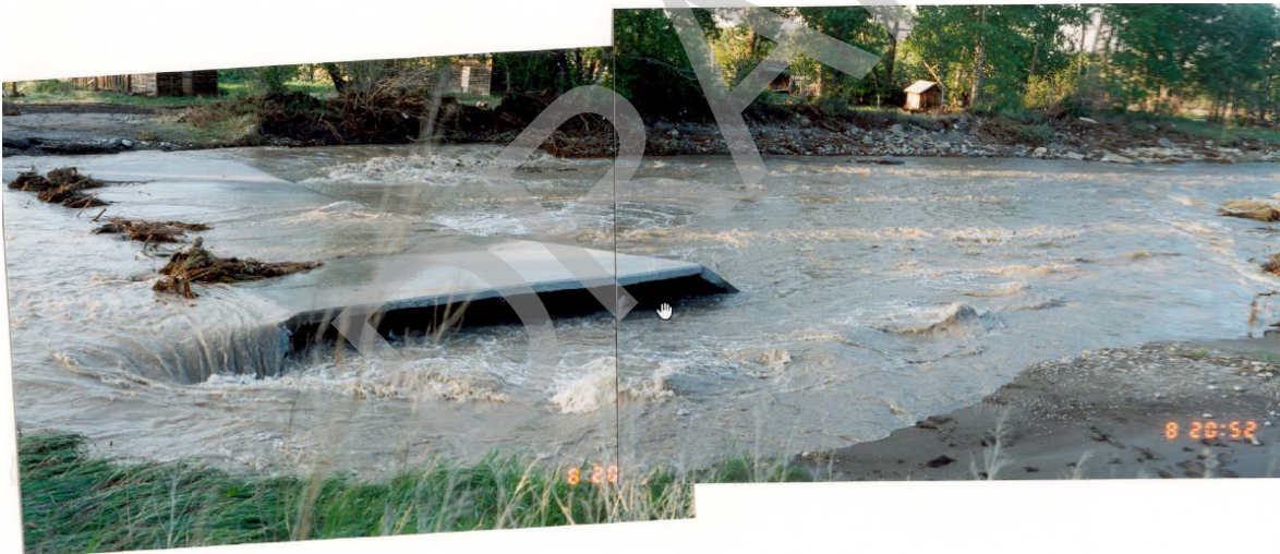
Figure IV.8 Washout of the Low Level Crossing upstream of the Kettles Creek Confluence
