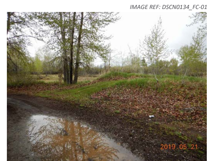
3. View looking at the downstream end of the berm toward the creek (on the other side of the flood control structure).
