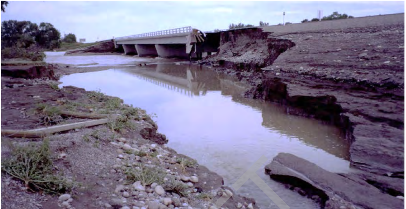
Photo 1 Highway 2 erosion of right abutment, 1995 flood, north facing view (Alberta Transportation, 1995)
