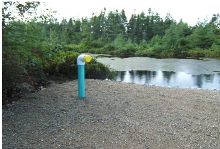
Figure 1.7 Dry Hydrant - An example of a dry hydrant installed on a pond with gravel surface off main road for access. See detailed example in Appendix F
