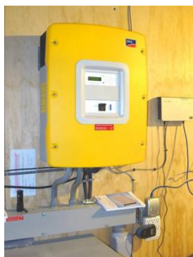
Figure 6 – Inverter panel – Photo credit – Sunny Island
