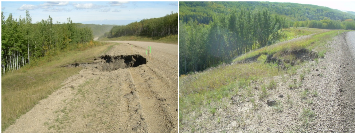
Figure 1: Typical Slides along Existing Highway 727 Requiring Repair
