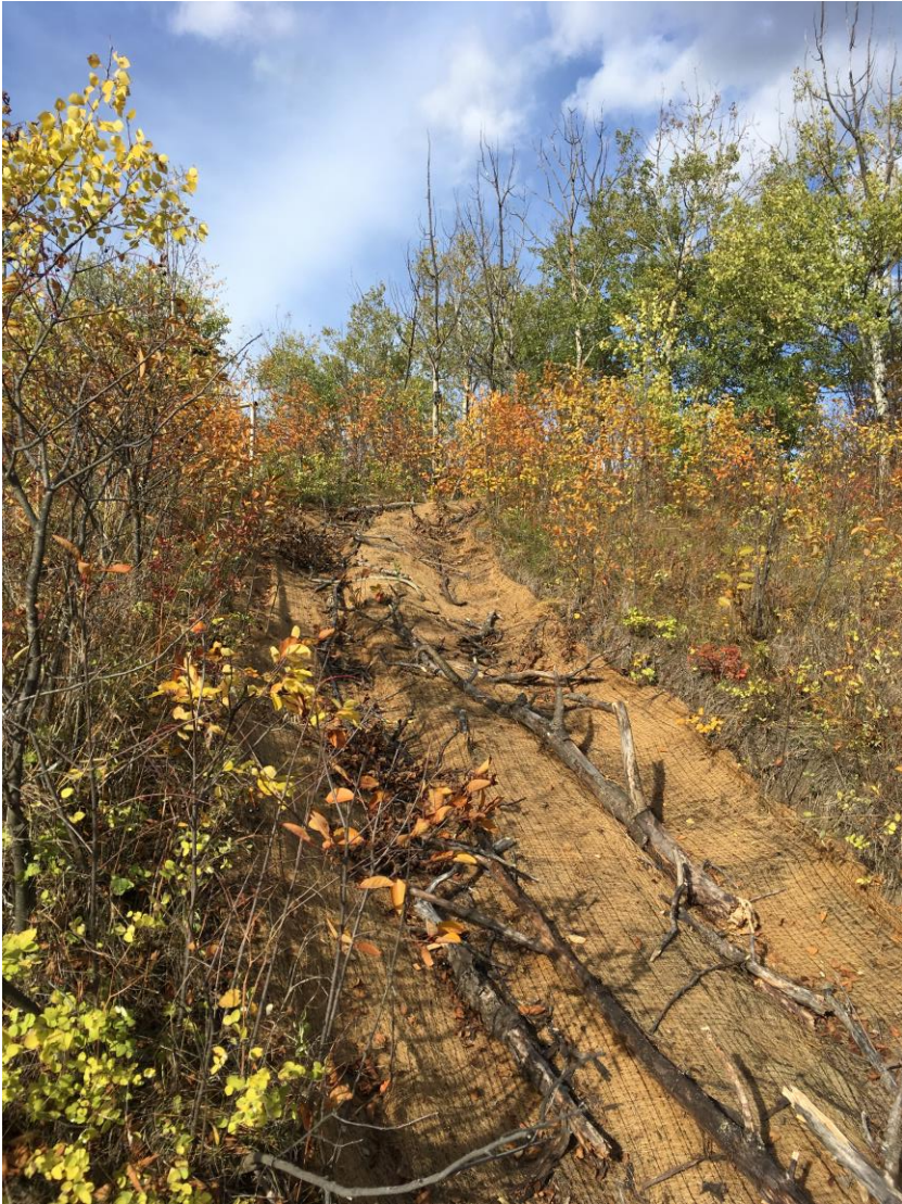
Figure 10. Erosion control blanket and woody debris on old trail (looking up from part way down the slope)
