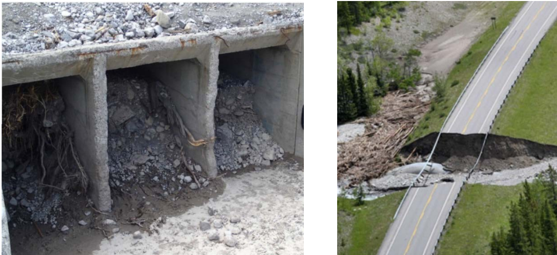
Figures 5 and 6: Culvert Plugging (Cougar Creek, Highway 1) and Culvert Washout Conditions (Highway 40)
