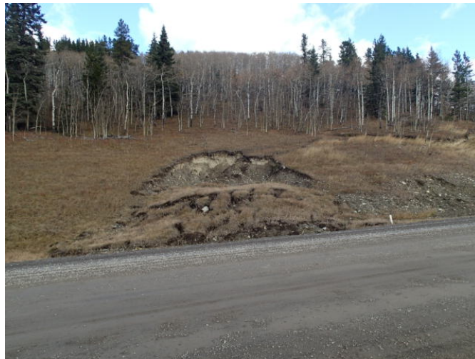
Figure 11: Example of Backslope Slip (Highway 68)
