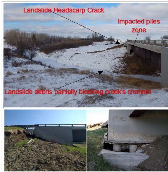
Figure 2. Landslide Features (2017 and 2018)
