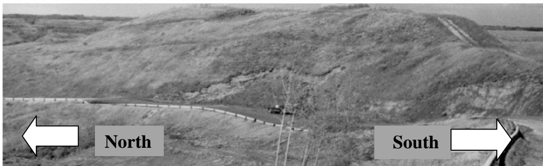
FIG.4. Vertical Drop in Roadway and Backslope Michelin Slide - North
