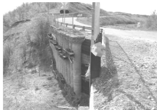
FIG. 13. CNR Slide, May 13, 2013 25 years after Stabilization
