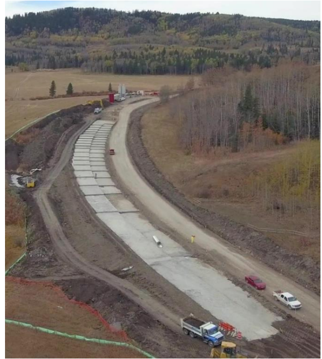
Figure 9. Photo showing completed placement of cellular concrete prior to backfill with granular
