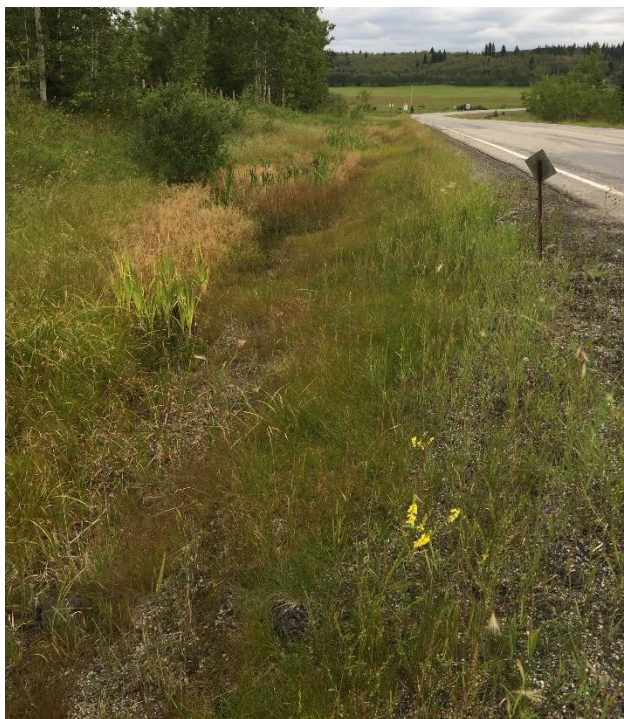
Figure 4. Photo of poorly drained area on NW side of roadway looking NE, August 2016
