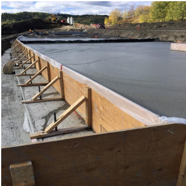
Figure 8. Photo of wood formwork on sides of cellular concrete, and transverse nonwoven geotextile partitions
