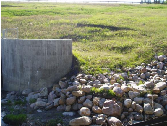
Figure 1. General view of the south slump.
