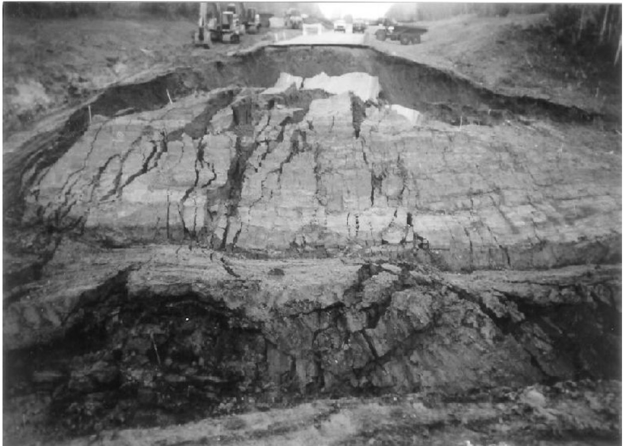
Figure 2: Excavation Slope Failure, Hwy 88 Culvert Replacement Project
