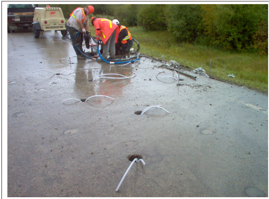
Photo 4. Finished installing confinement unit and hose into borehole. Workers attaching tremie hoses to foam guns.
