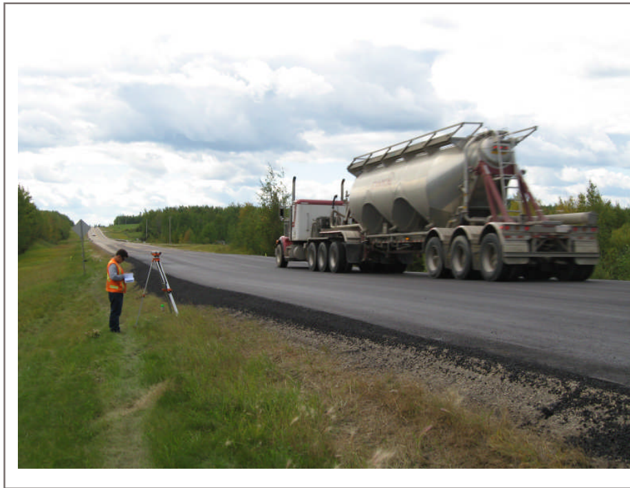
Photo 8. Looking south. Re-establishing the survey points after the asphalt overlay was placed
