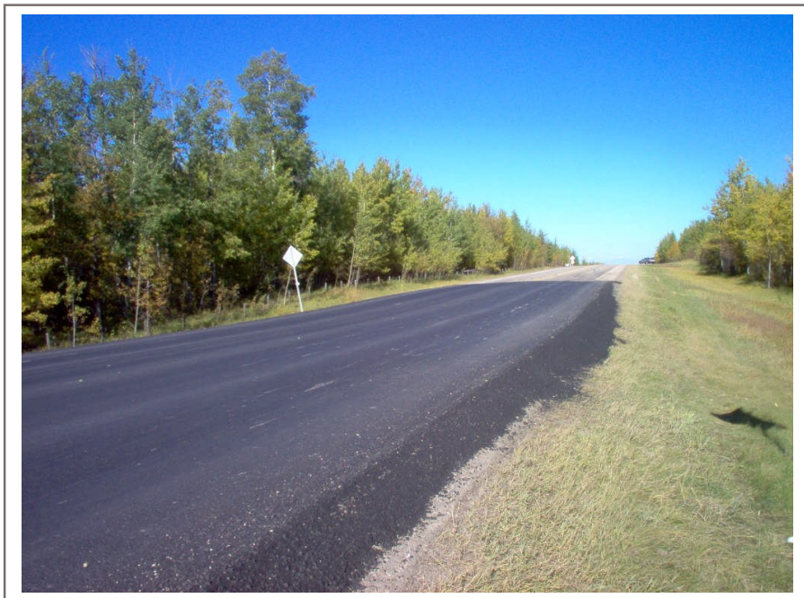
Photo 7. Site after asphalt paving to reprofile dip in the roadway, looking north
