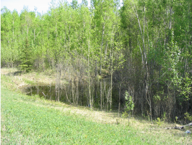
Figure 1. Pooled water in south ditch at blocked culvert location.
