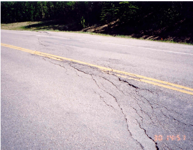
Figure 2. Pavement distress, west flank of the slide, looking southeast.
