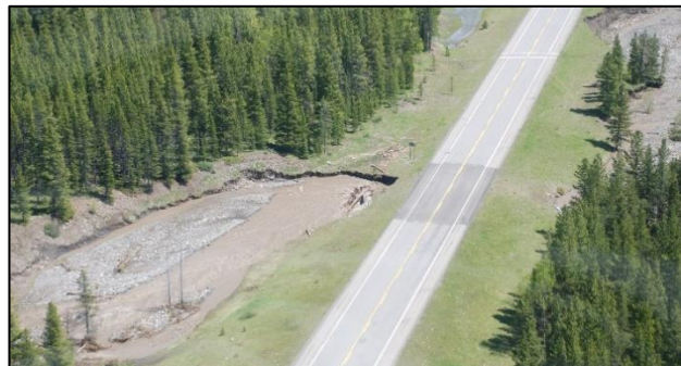
Figure 3. Highway culvert erosion hazard (AT image).
