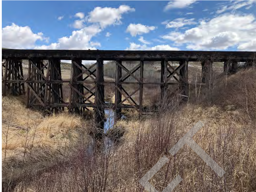
Camrose Creek (downstream view) at the CN Railway Trussell Bridge near River Station 1,485 m.
