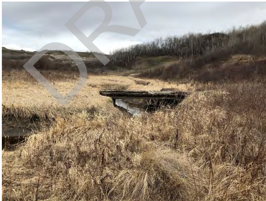
Camrose Creek (upstream view) at a Trail Bridge near River Station 720 m.
